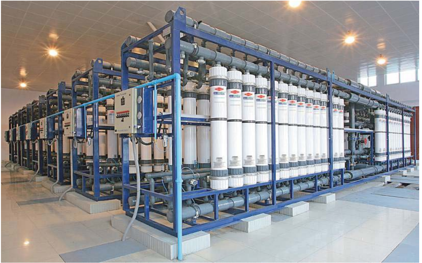
Figure 9: DOW UF Installation using 2860 Modules
